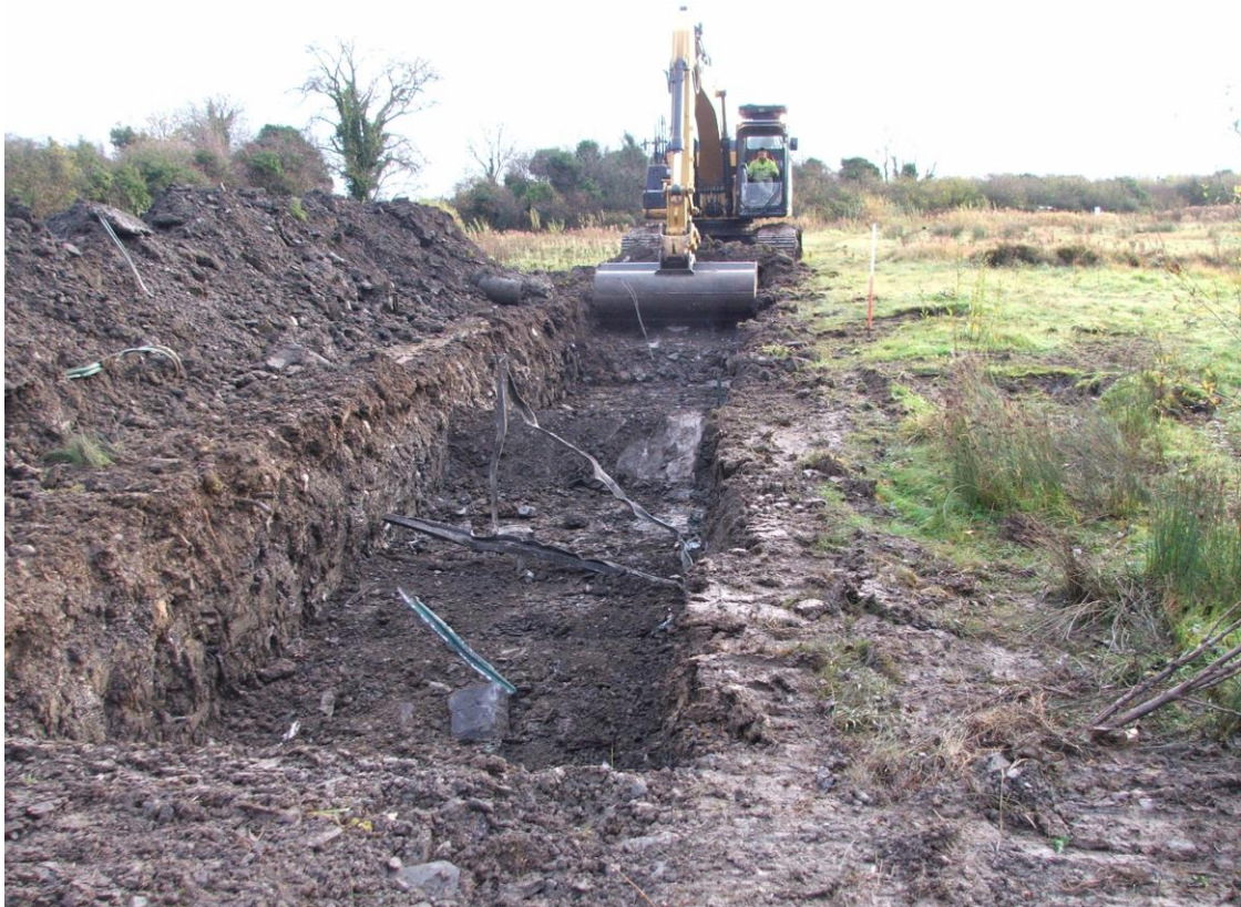
Plate 2: Modern disturbance in Field 1 Trench 5
