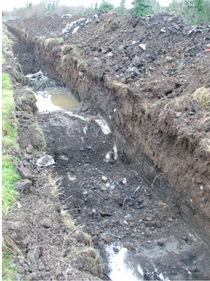
Plate 9: Modern disturbance in Field 4 Trench 2
